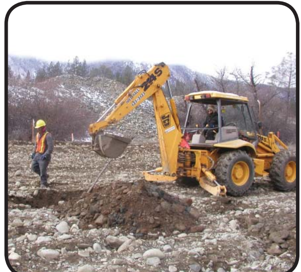
Using backhoe to dig 10-foot deep planting holes so live stake cutting contact groundwater.
