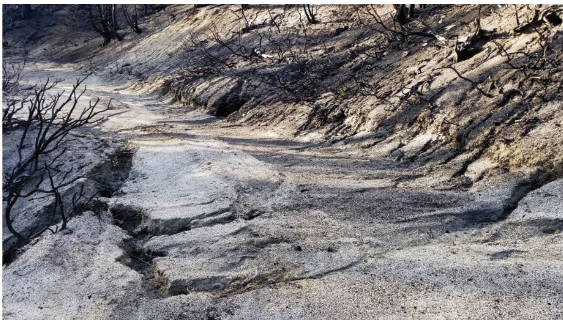
Rill and gully erosion causing road fill failures on Mainline Spur A Road
