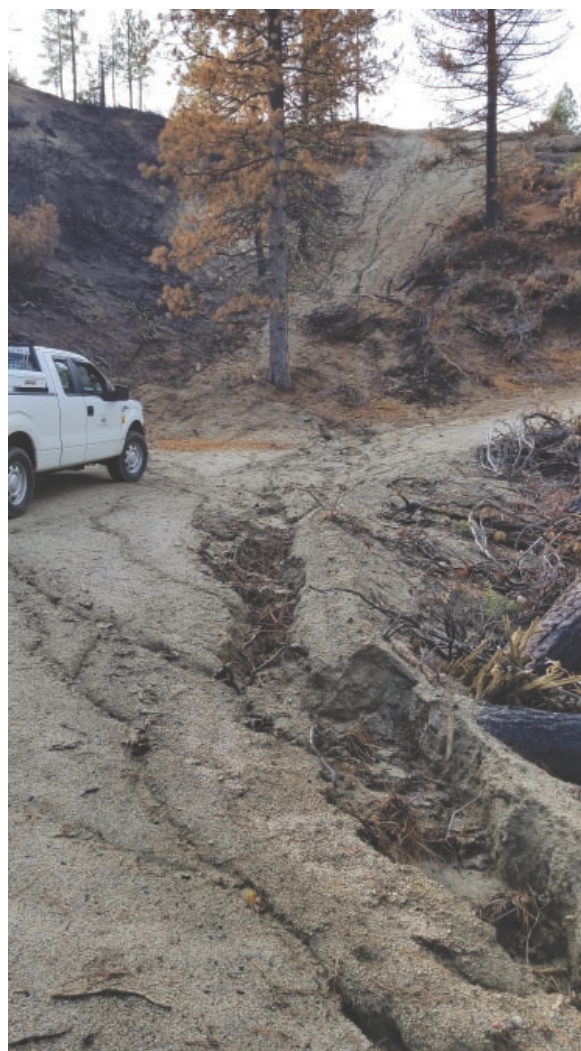
Rill and gully erosion on Mainline Road
