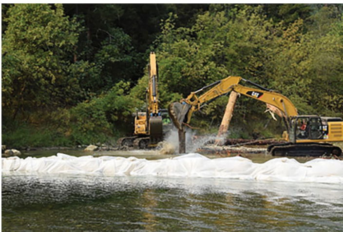
Figure 5. Logs are keyed into the river and overlaid with additional logs and boulders.
