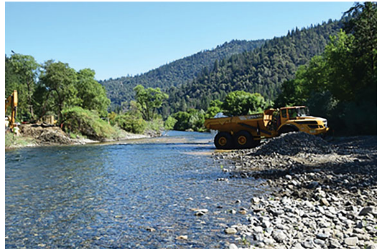
Figure 1. In-river construction work at the Dutch Creek project site on the Trinity River began on July 15
