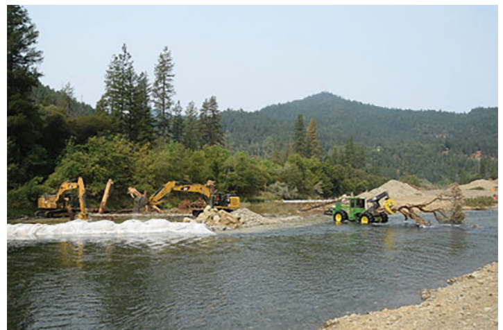
Figure 6. Dozens of whole trees are used during the construction of the logjam.
